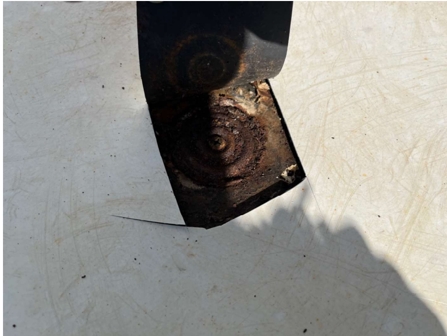
Overview of corroded fastener and plate in mechanically attached roofs.
