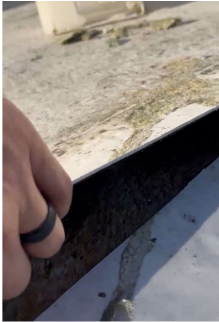
Close view of membrane delamination from LWIC.
